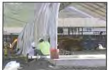
One emergency transitional shelter has opened at Kalaeloa, and a second is being constructed in Wai'anae by
