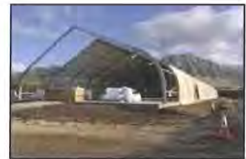
This temporary homeless shelter is taking shape in Wai'anae. Metcalf Construction is building the sprung structure ? it will be 70 feet wide, 270 feet long ? in a lot near Wai'anae Intermediate School.
